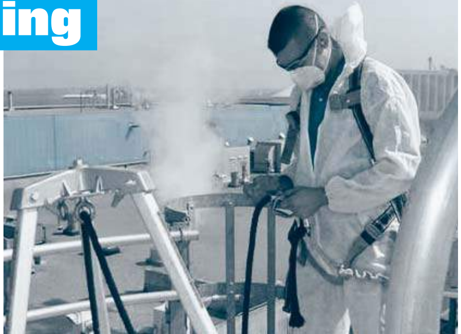
Familiarity with full protection equipment is essential to bin cleaning procedures.
