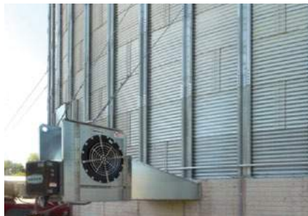
Grain temperature control is the key tool to non-chemical insect control in stored grain.
